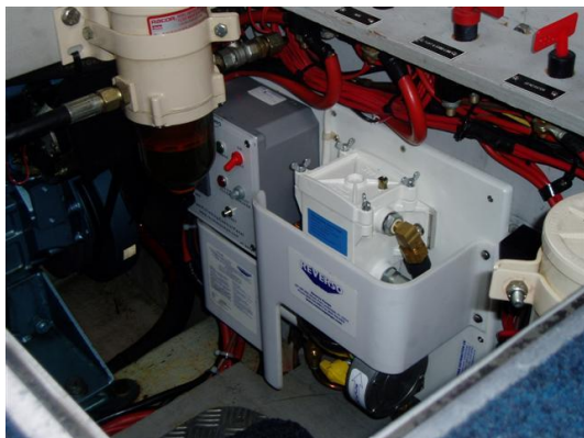
The fuel polishing installation
