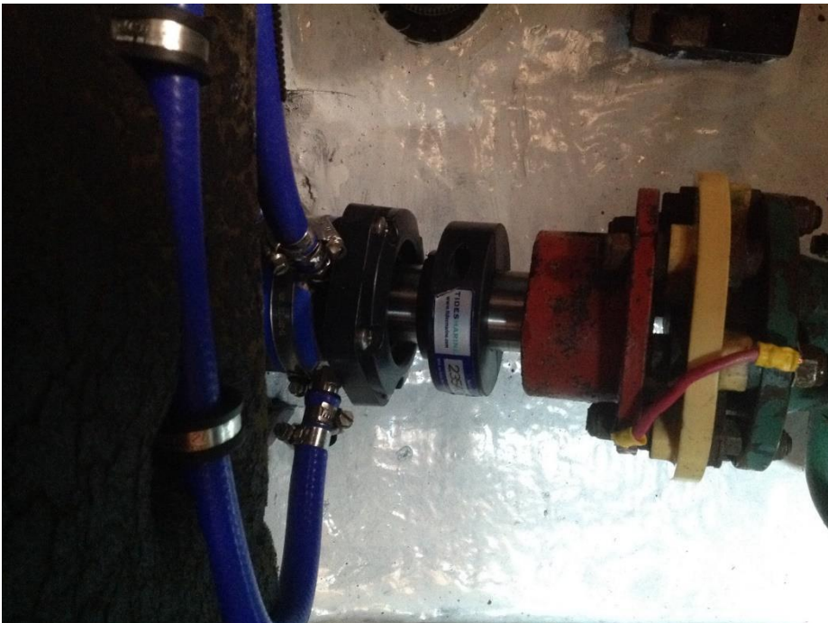
The finished assembly with new shaft, seal and the spare seal mounted in the black collar between the seal housing and the coupling flange.
