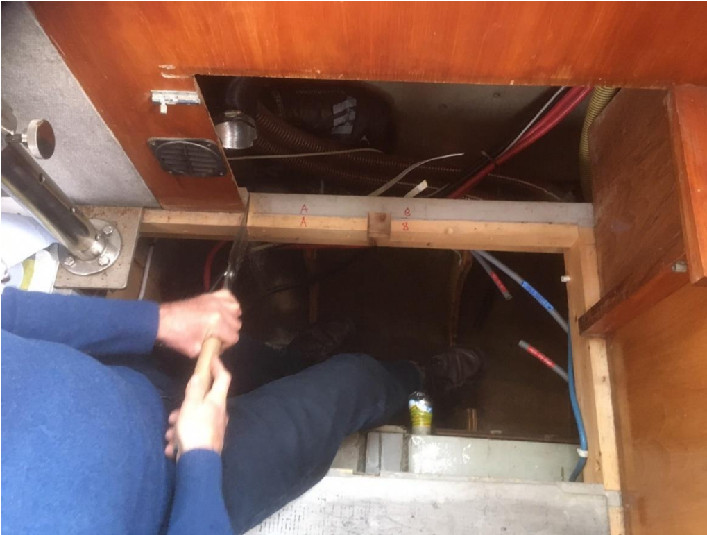
Cutting through the beam to allow fitting of the new 14" diameter calorifier.
